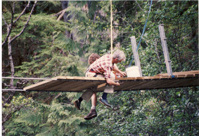
Building the Gayle McGee suspension bridge on the Bedwell Trail in 1998. Walter Latter putting on the deck and stanchions.
