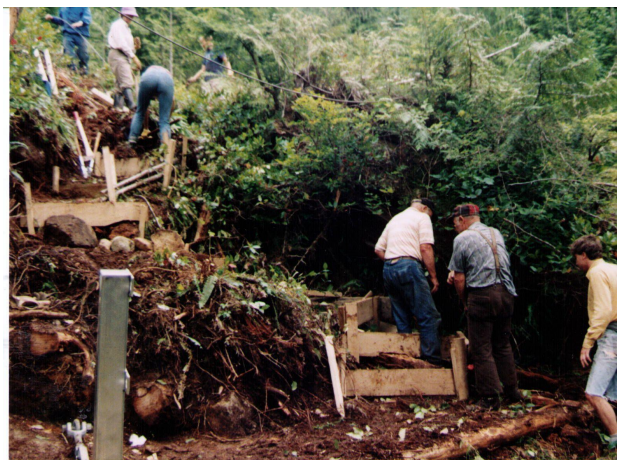
Working on the approach to the Gayle McGee Bridge. Stan and George Doran are front and center working on some stairs.
